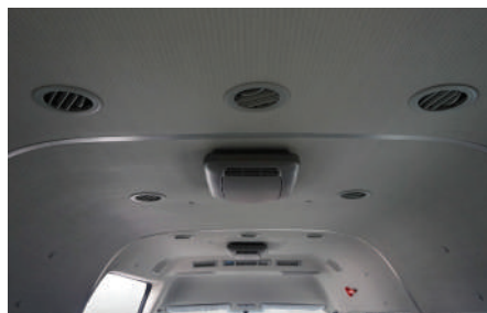
DOUBLE REAR A/C UNIT WITH 9 ROOF VENTS
