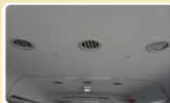
Rear A/C Unit with 6 Roof Vents
